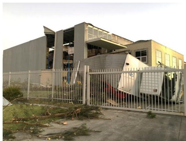
Figure 5 Damage to industrial building on Chisholm Road, Kurnell, with overturned truck in foreground.
