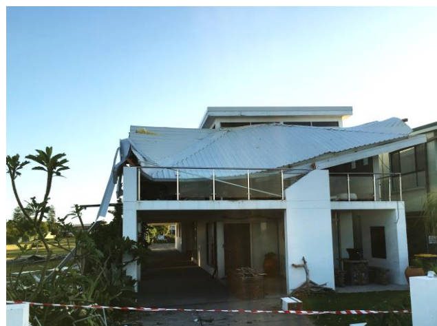
Figure 6: Damage to a residential home in the Kurnell township.
