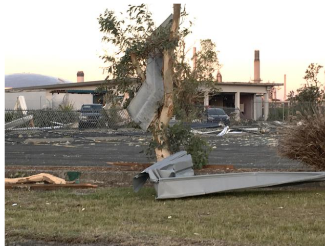
Figure 4: Debris from the desalination plant and other surrounding buildings on Sir Joseph Banks Drive, Kurnell.
